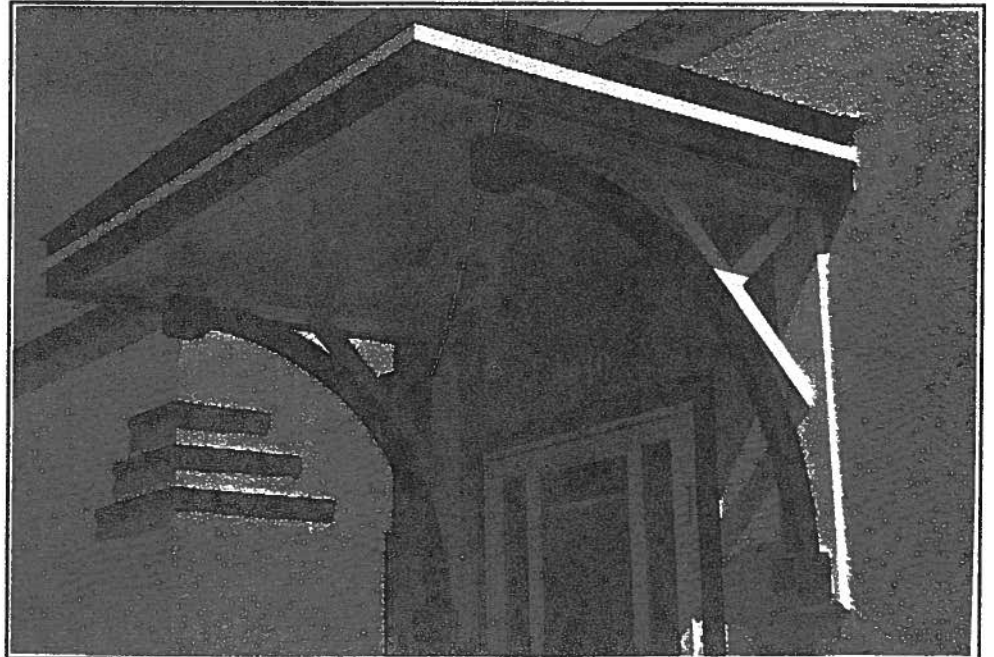
Fig. 19 Painted wood canopy and brackets on Dr. Carroll's residences after restora- tion
